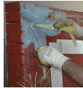
Inserting the FRP anchors into the predrilled holes over the last layer of polyurea
